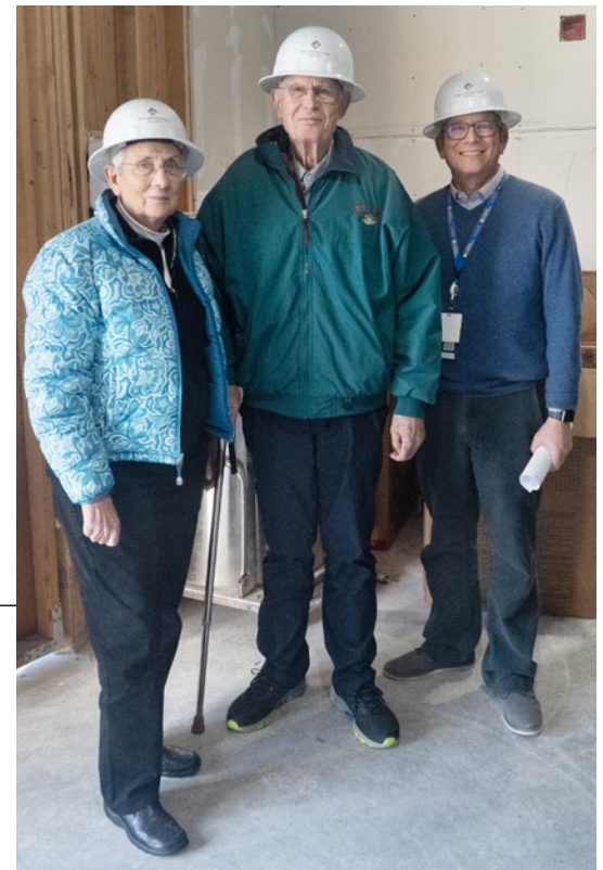
From left, Dmarlou Foundation trustees Susan and Richard Rahl with CCAH Director Michael Kent as they tour the new Advanced Veterinary Surgery Center under construction. Photo: Mike Bannasch
